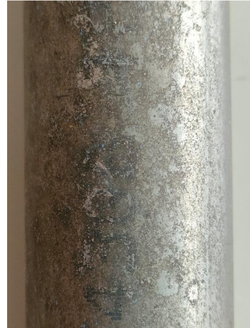
Steel pipe: rough, partially rusted
